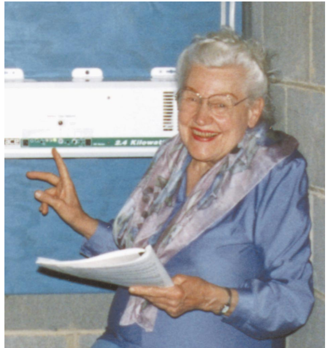
Above: Jane Sharp checks out the owner's manual for her new Trace 2424 inverter.
